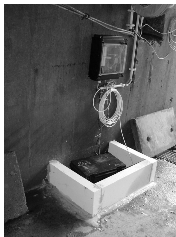
Figure 5 : Accelerometer ETNA installed at the Membach station in 2003
